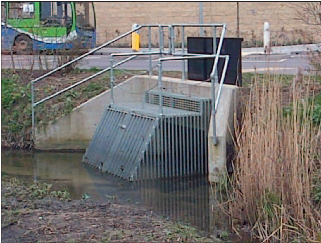
Figure 3: River Bure trash screen at Hanover Gardens during normal flows looking east
